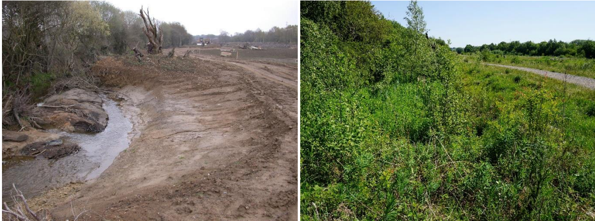
Fig 5 (left) 15 th April 2016, illustrates the works undertaken to de-canalise Hawke Brook. On this section banks slopes were reduced, the width was increased and a second channel formed to accommodate flood waters and allow them to lose energy and deposit silts.
