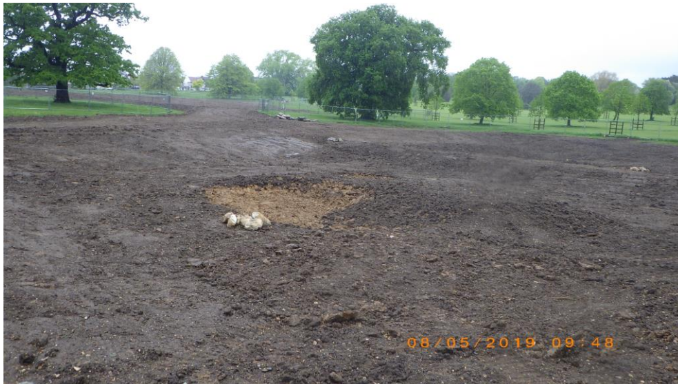
Final shaping of wetland cells with topsoil including formation of bund, deep pools and islands (early May 2019)
