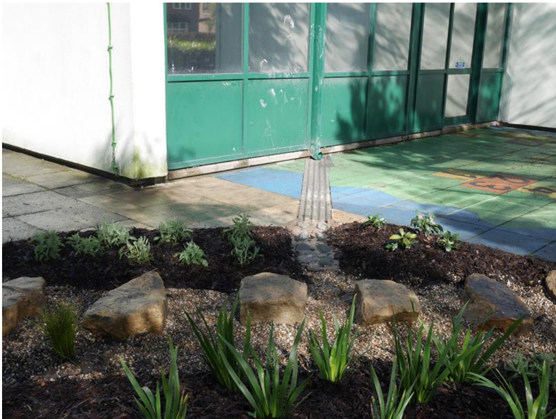
Fig 3: Fluted drain and river washed cobble cascade transfer surface water to the raingardens
