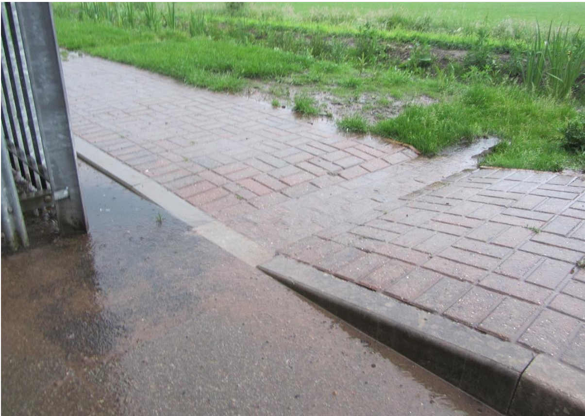
Fig 5: Wetland Swale Drop Kerb Inlet Year 1
