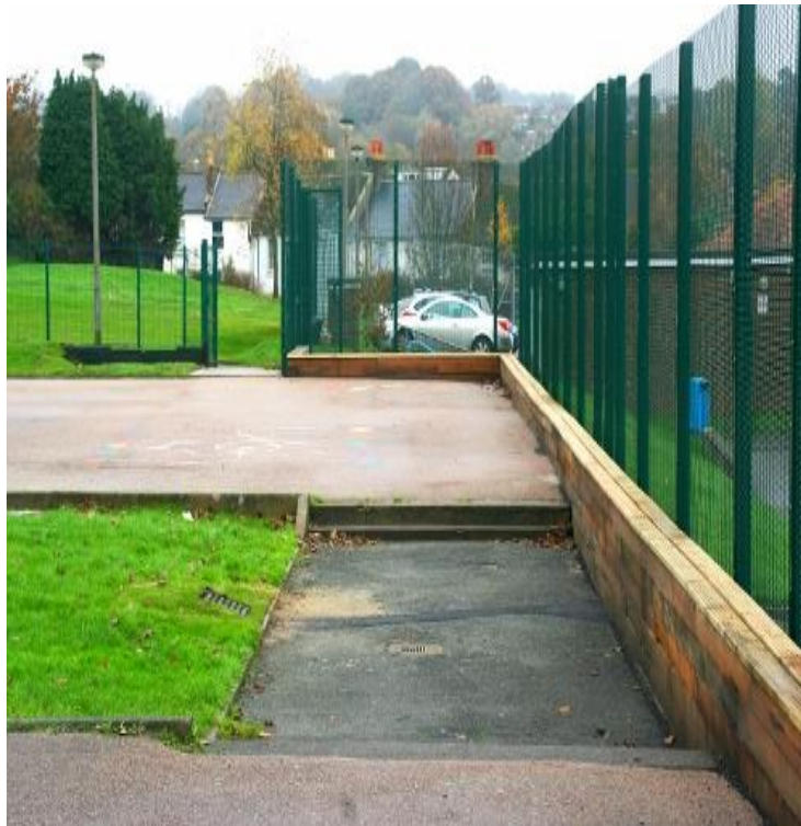
Figure 3 Timber seating wall converts an existing hard play area into a water large storage facility whilst providing added amenity for children
