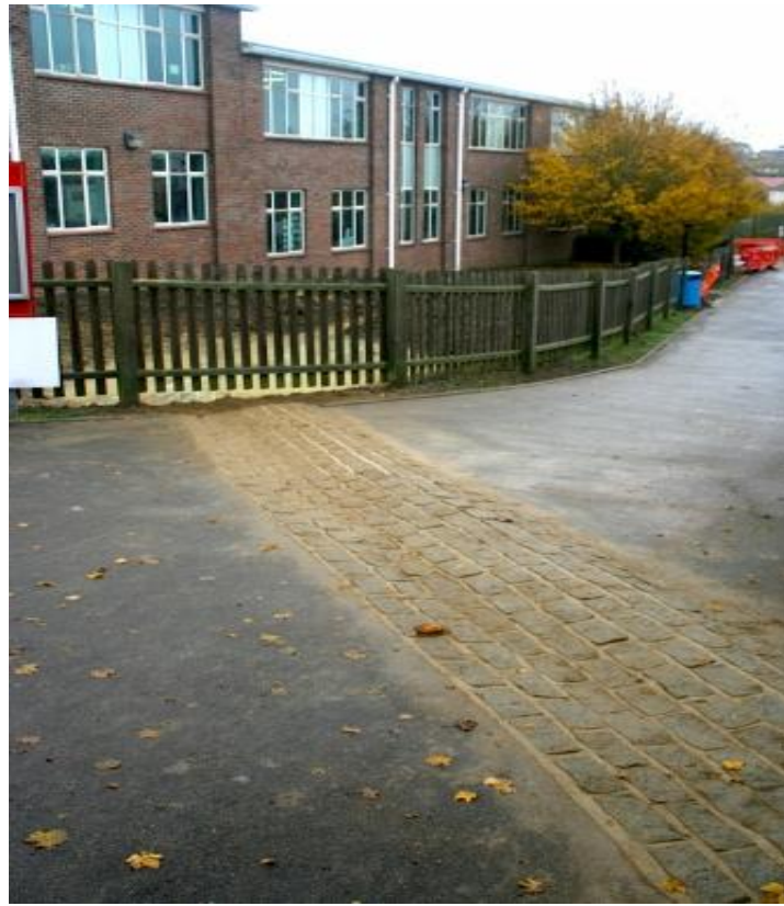
Figure 4 Granite sett flow diverter comprising combined channel and hump in a wave-like formation. The channel intercepts overland flow and diverts it to the raingarden basins beyond the fence (shown during construction)
