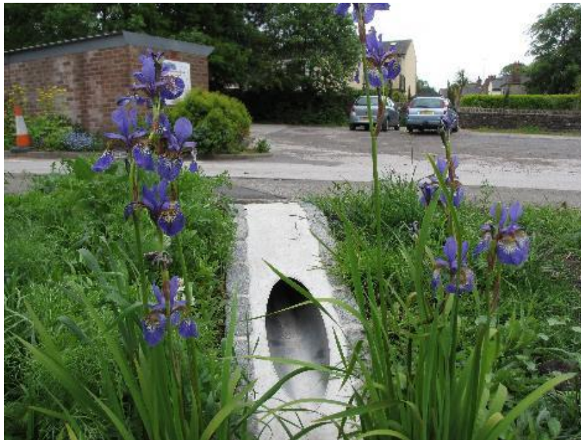
Figure 7 The headwall is mitred, with stainless steel inlet pipe and granite sett surround into the short swale
