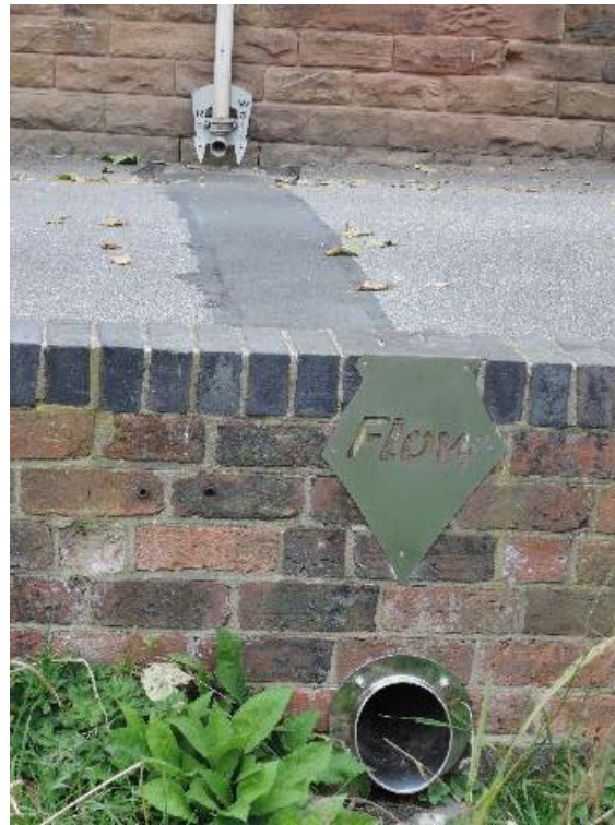
Figure 15 Disconnected downpipe which was diverted to an underground pipe due to the reverse fall to the raingarden. Note interpretation and stainless steel spout inlet
