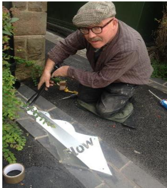
Figure 14 Artist Richard Bett creating stainless steel interpretation of the SuDS management train throughout the site, complementing the stainless steel detailing of the features
