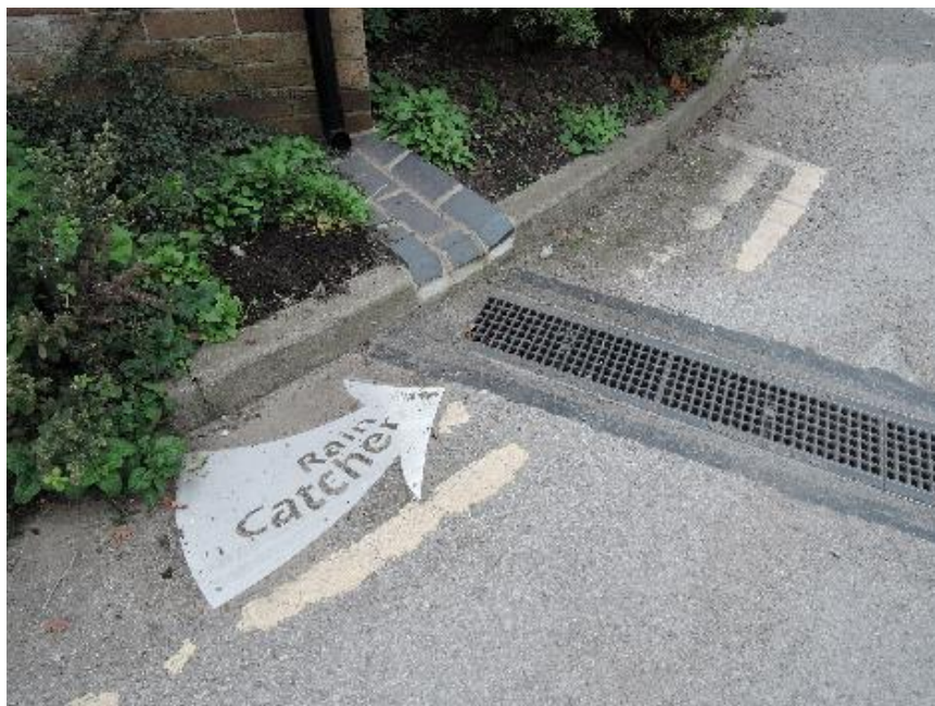
Figure 16 Raincatcher' grating, originally specified as stainless steel but the tight budget unfortunately meant a more conventional finish. Dowbpipe is from a small shed
