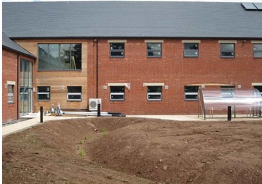
Figure 7 The swales were graded to be very shallow to enable mowing (During construction)
