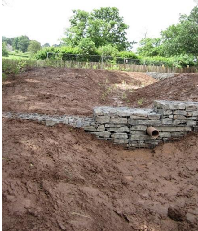
Figure 6 The treatment train of open swales and wetlands, separated by gabion baskets, filtering and infiltrating the water before discharging into the brook (During construction)
