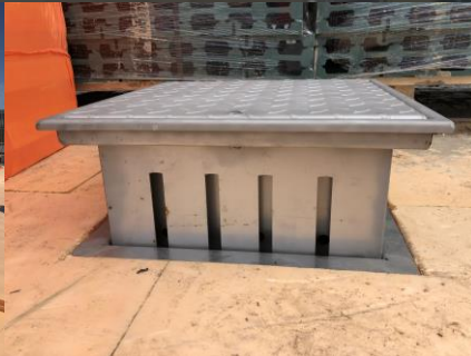
Restrictor chamber Level 60
