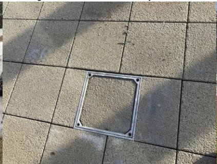
Level 50 chamber lid recessed into paving
