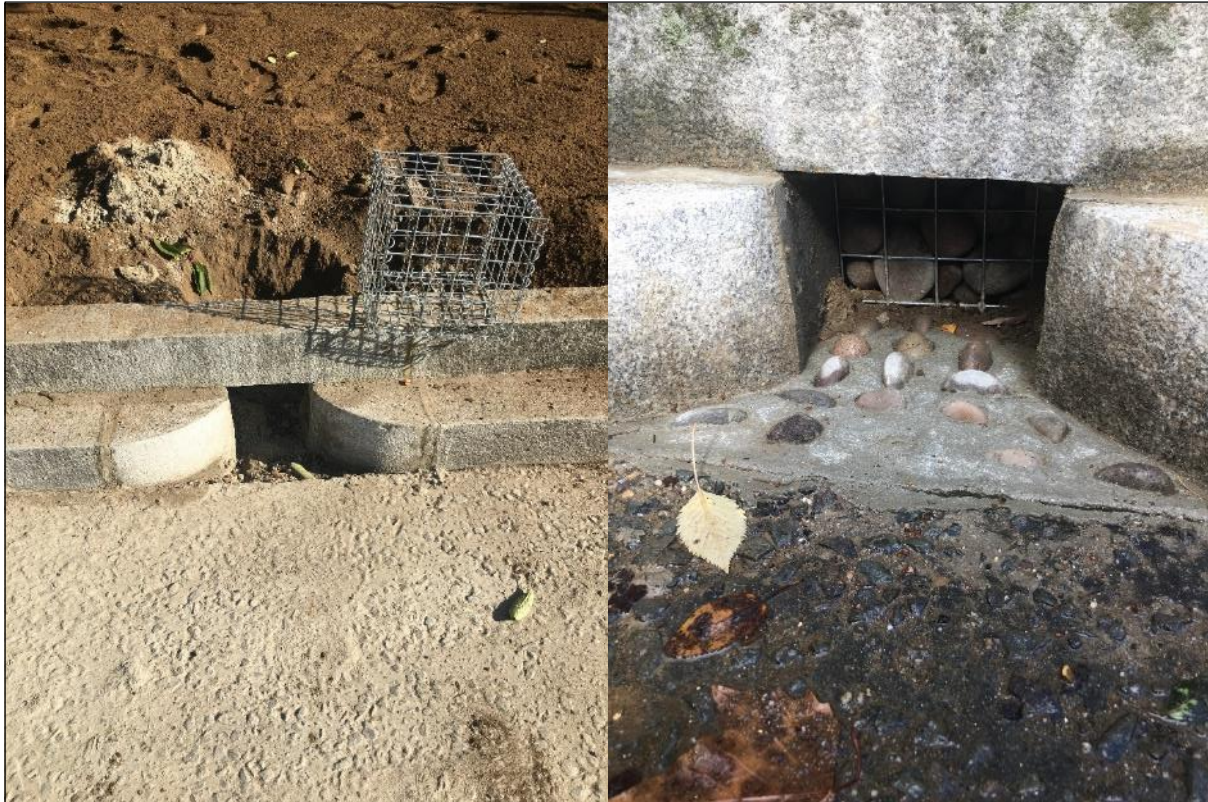
Figure 4: Gabion basket kerb inlets
