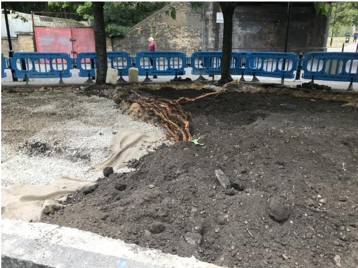
Figure 6: rain garden during construction. Crushed aggregate sub base overlain by hessian and soil.
