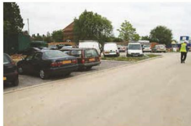
Figure 12.2 Sacrificial sub-base layer allows use of permeable sub-base for parking during construction
