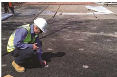
This process prevents mud/site material blocking the permeable base. It is then filled with granular material to allow drainage, before final permeable finish
