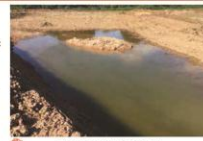
Using SuDS basin to collect silt
