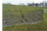
Soil washed down slope, creating flow channels
