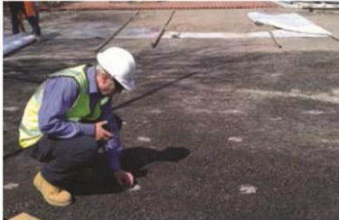
This process prevents mud/site material blocking the permeable base. It is then filled with granular material to allow drainage, before final permeable finish
