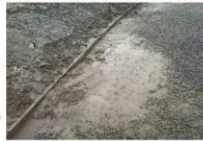
Washout from banks causing silt build up on paths
