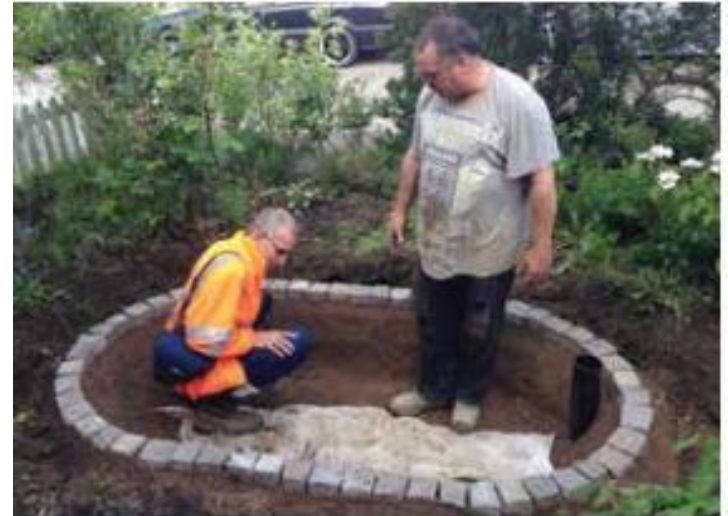
Unlined rain garden on clay soils provided with outfall connection
