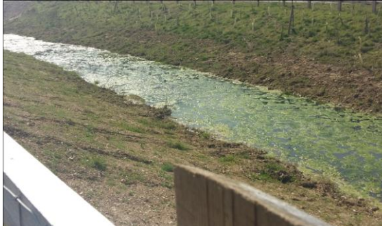
A blockage has resulted in standing water which has developed an algal bloom. The sides of the swales are not correctly planted
