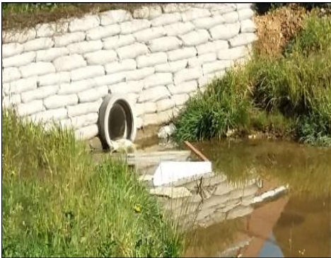
Rubbish could create blockages
