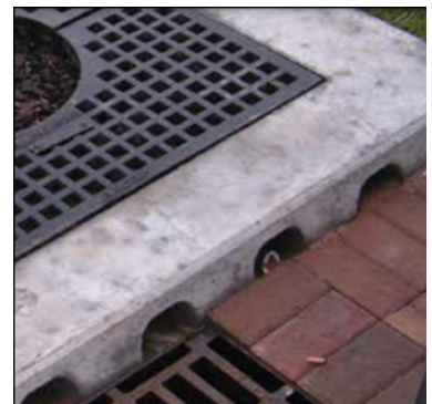
Outlets blocked by other features
