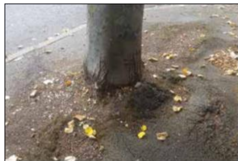
Tarmac around a tree whose roots are pushing up the surface of the pavement.
