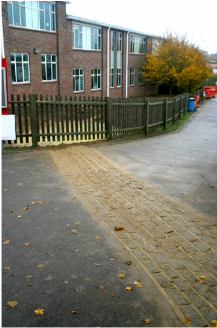
Figure 4: Granite sett flow diverter comprising combined channel and hump in a wave-like formation. The channel intercepts overland flow and diverts it to the raingarden basins beyond the fence (shown during construction).
